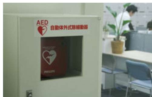
Installed near workplaces and accessible in case of emergency
